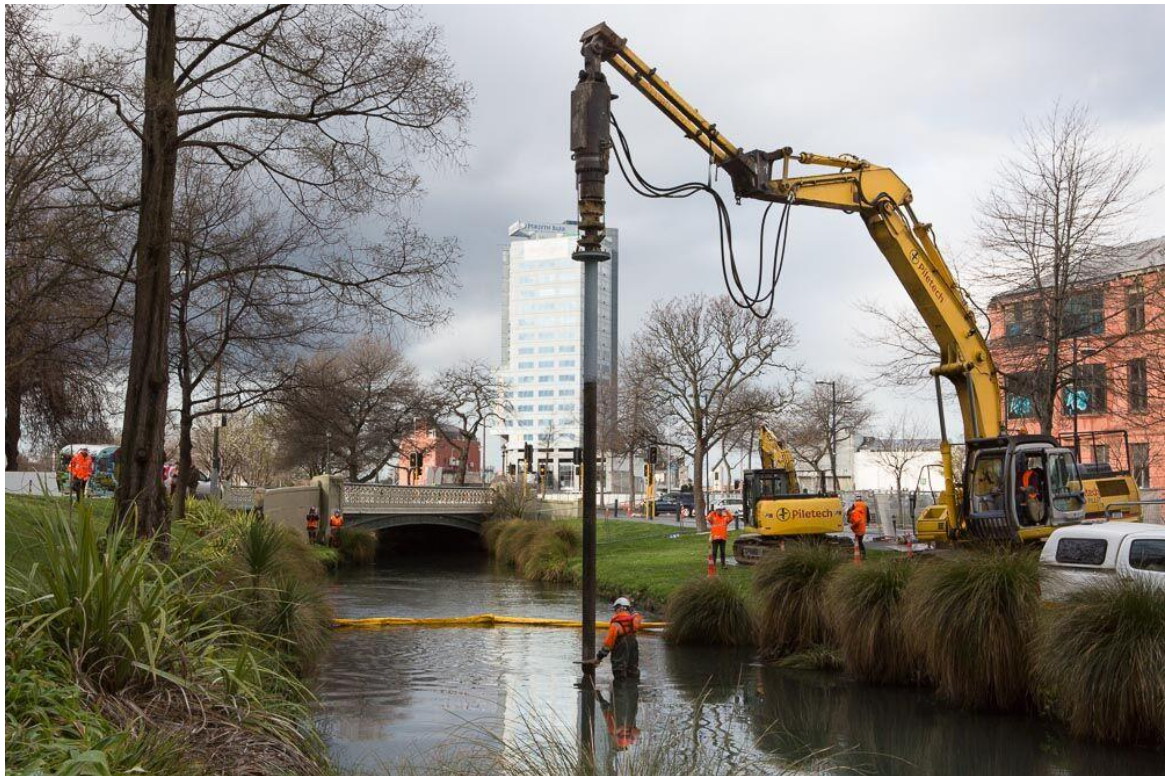
The team from Piletech working on foundations for the Gormley sculpture in the Avon River Christchurch.
