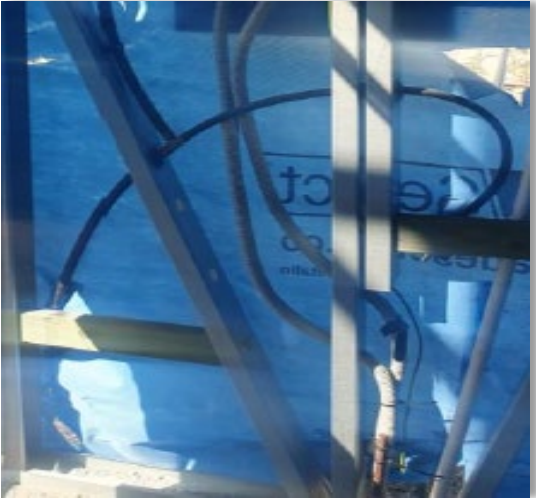
While tight bends are still visible in these images, the pipes are able to freely expand and contract within the open wall cavity during expected regular changes in the pipe's temperature and pressure (e.g. water hammer).
