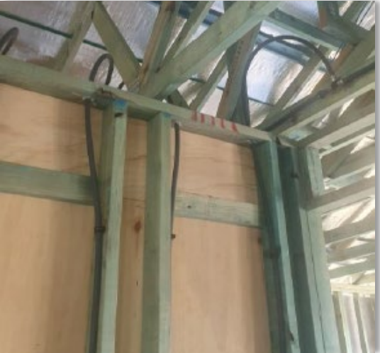
Holes cored in the top plate allow for adequate movement of the pipe due to thermal expansion and contraction without being held tightly by a mortar fill.
