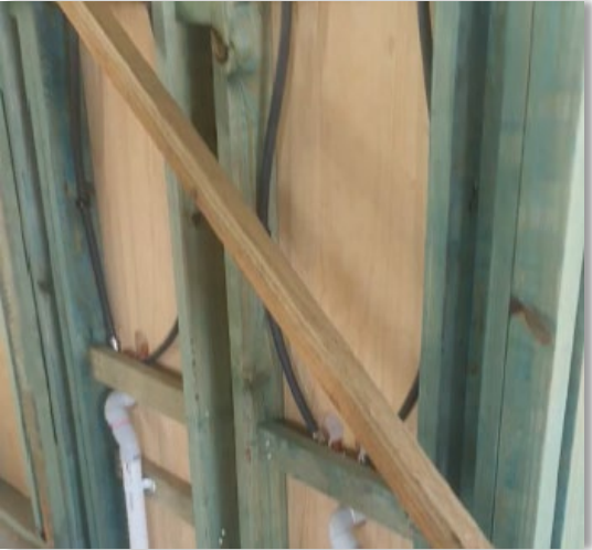
Timber frames allow the pipe to be installed within the open space of the wall cavity, allowing for adequate movement due to thermal expansion and contraction , while still being supported with sufficient clipping.
