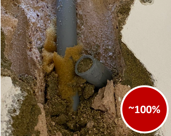
Lagging not impermeable (and at times non-existent)
