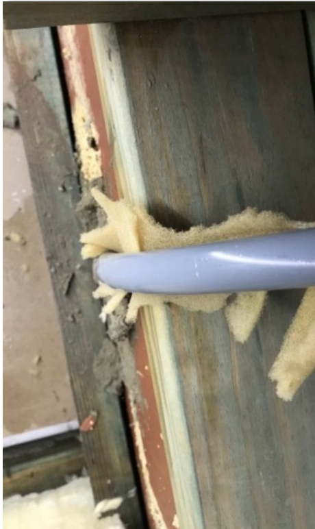
Pulled hard against timber not allowing for lineal thermal expansion per guidelines
