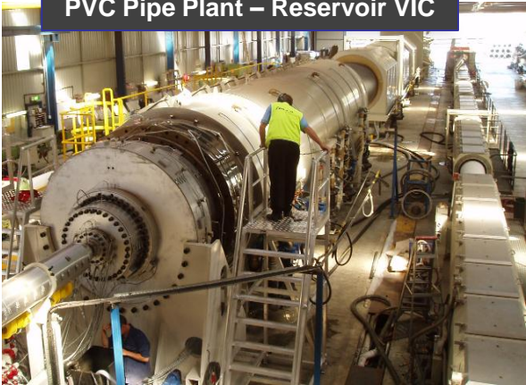
PVC Pipe Plant – Reservoir VIC
