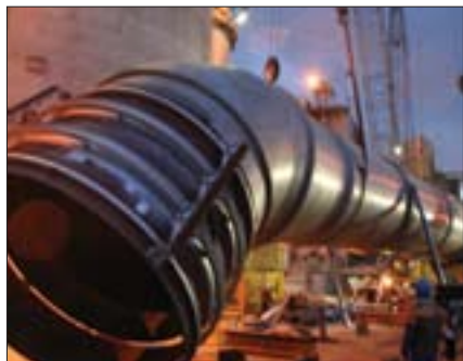
Gas ducting being lifted into place as part of the Gas Train Modification project at the Golden Bay Cement plant near Whangarei, New Zealand.
