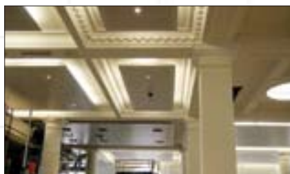
Specialist metal ceilings installed by Forman Commercial Interiors at the Britomart transport project, in Auckland, New Zealand.
