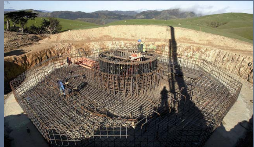
48 tonnes of steel in each 15m base of the 112m high Makara turbines
